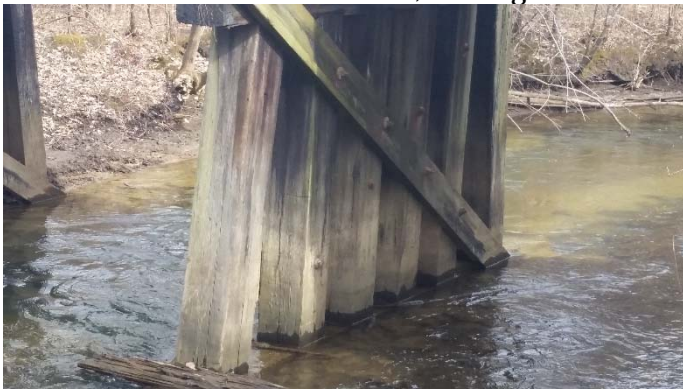
Close-up of the middle timber piles Taken from the west side, looking east
