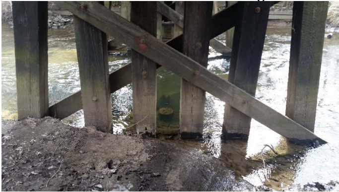
Close-up of the 3 rd support piles and erosion Taken from the north side, looking south
