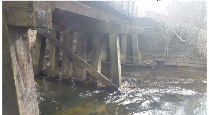
Close-up of the 3 rd , 4 th , and 5 th support piles Taken from the Northwest side looking southeast
