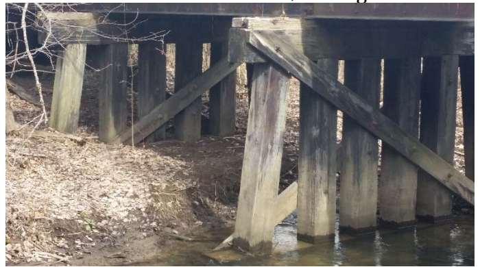
Close-up of the northern two support piles Taken from the west side, looking east
